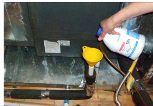
HVAC drain line by furnace in attic
