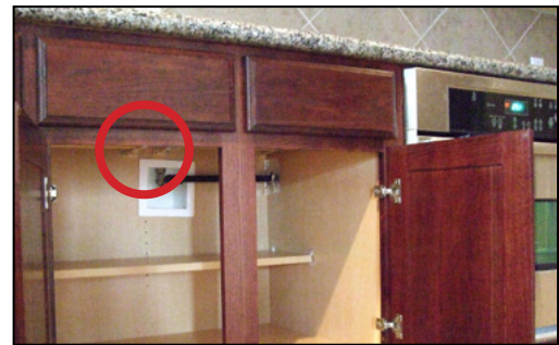
Gas shut off valve
