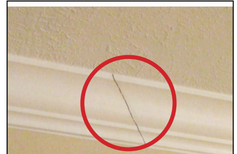
Interior trim crack
